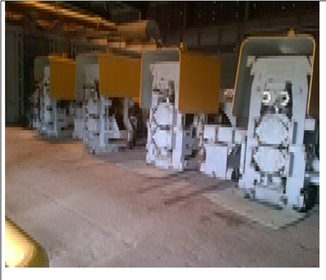
Plate 3.2: Exit end of Reheating Furnace and The Roughing Mill.
