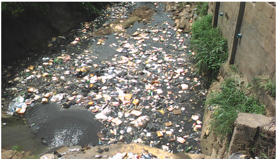
Refuse dumped in adrainage along Farayola Street, New Bodija, Ibadan.
