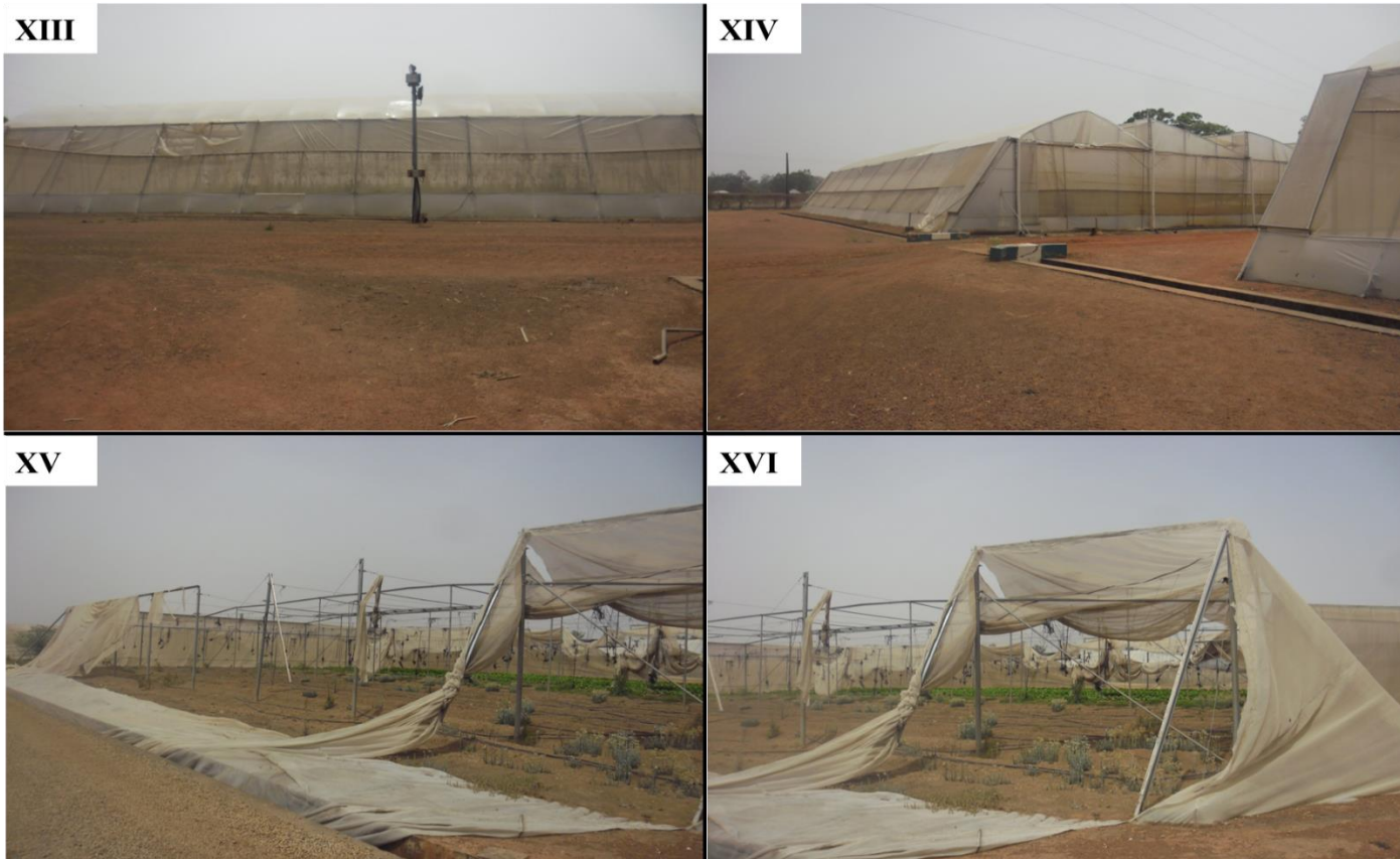
HIGH COST GREENHOUSES AT ASTC PLATEAU STATE (XIII-XIV); HIGH-COST GREENHOUSE IN A DILAPIDATED AND ABANDONED CONDITION AT ASTC PLATEAU STATE (XV-XVI)
