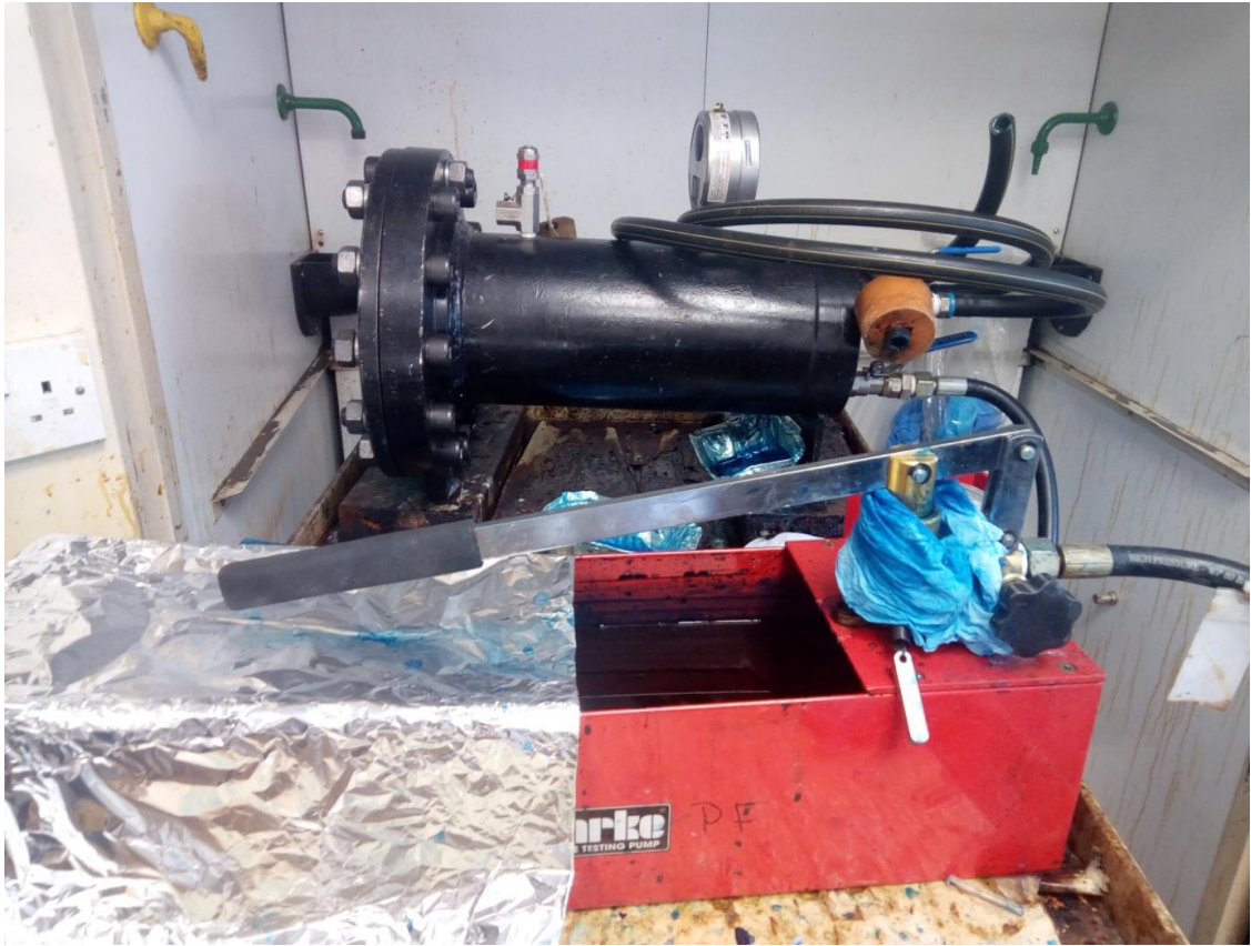
Plate 3.2: Pressure impregnation vessel
